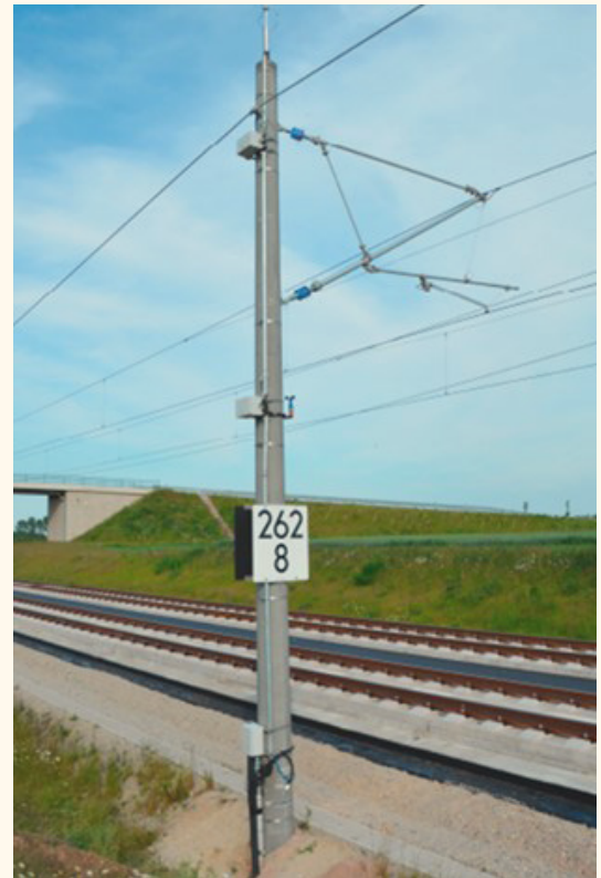
Fig. 2 The catenary pole system for high-speed rail routes.
